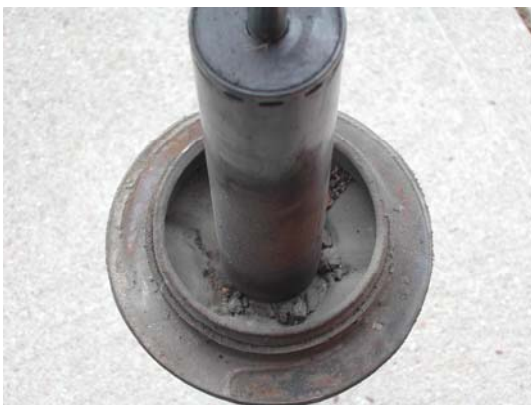
Typical accumulation of gunk - in this case some tar covered sticky gravel. All holes were blocked
